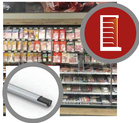
DOOR COOLER & FREEZER
